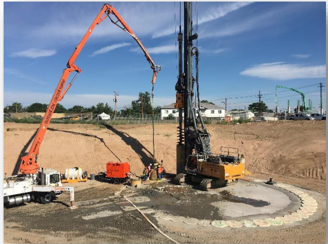
Pump station near York Street
